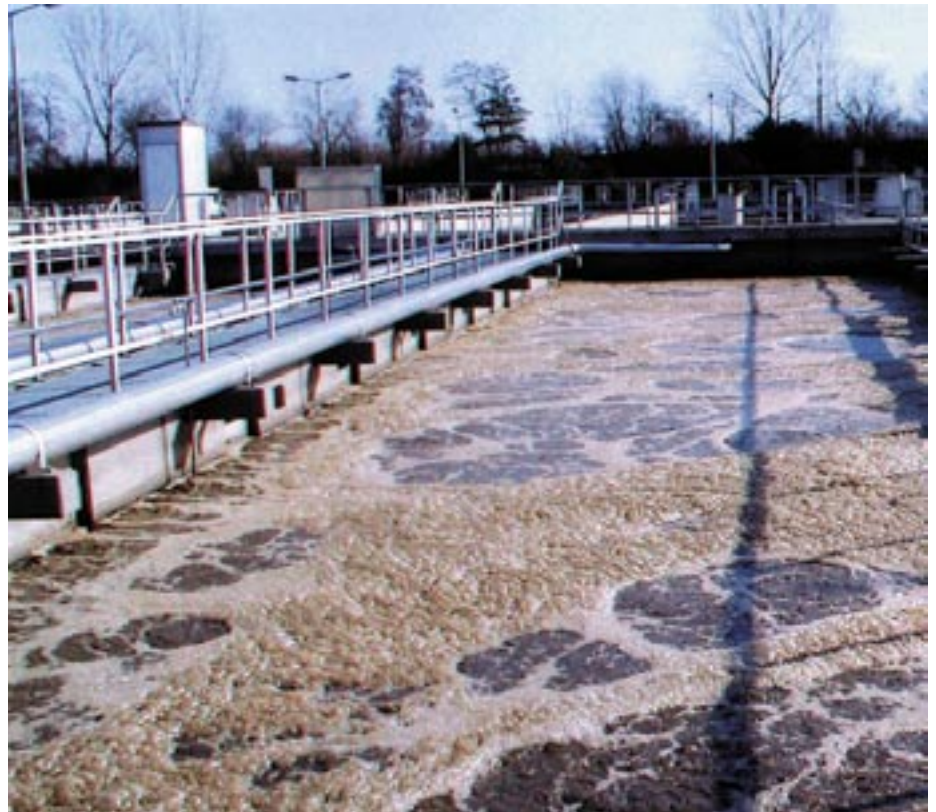
Figure 6: Aeration tank of a sewage plant. Fraunhofer IGB optimizes and expands the capacity of existing plants by systematic analysis and specific measurements.
