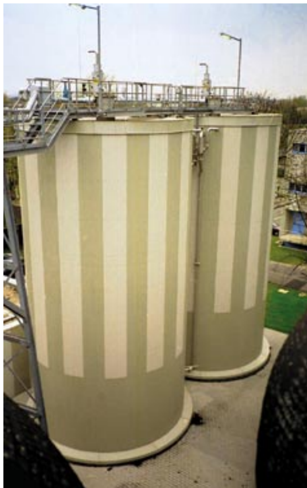
Figure 2: High-performance digestion installed upstream.
